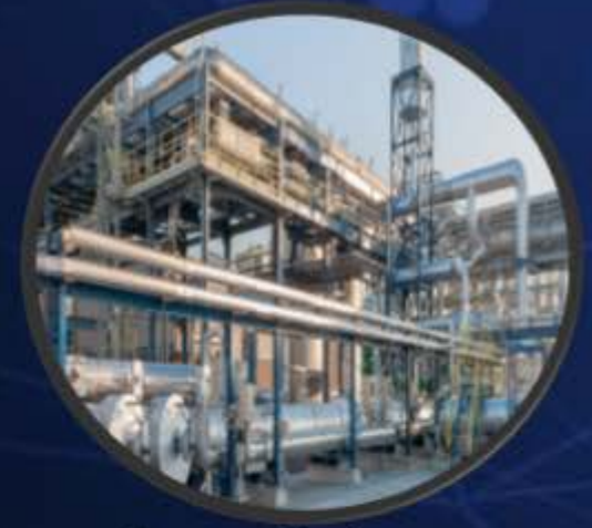
Green Hydrogen Production 100 – 250 MT/day Capacity
